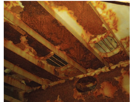
Poor tank condition
